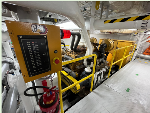
Generator Set Engine Room
