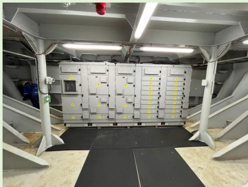
Operation Main Electrical Panel Engine Room
