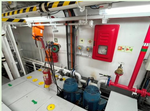
Fire and Black Water Pump Engine Room
