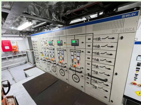
Main Electrical Panel 440V Engine Room
