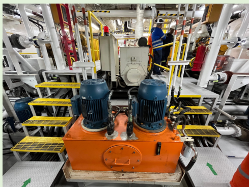
HPU Engine Room
